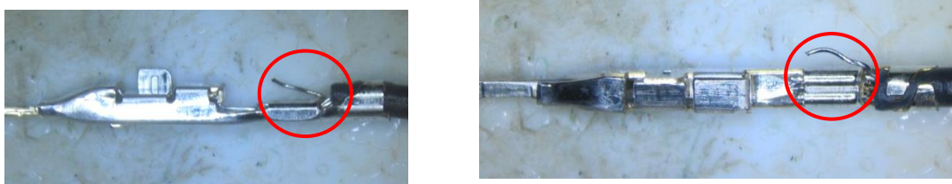
Fig 20. Incomplete conductors crimping
